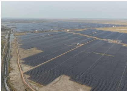
Dholera Solar Power Plant
